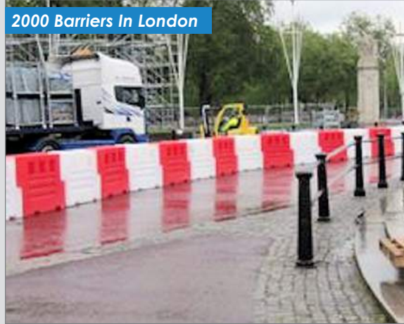
2000 Barrier Protecting Pedestrians
