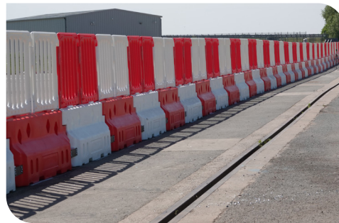
Installed with double top fencing
