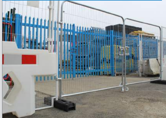
Vehicle Gate Used With Water Filled Barriers
