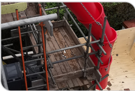
Rubbish Chutes connected
